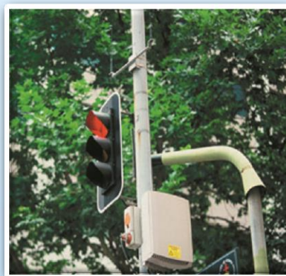
Microcell Mounted on Traffic Lights
