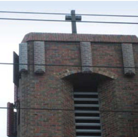
Antennas colour matched to the bricks of the church.
