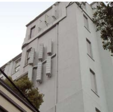
Antennas colour matched and flush mounted to an existing building.
