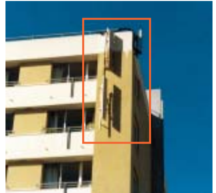
A better visual outcome may be achieved if the lower antenna were colour-matched like the one before.
