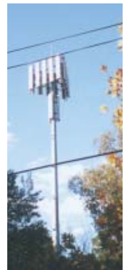
Flush mounted antennas co-located beneath a triangular headframe.
