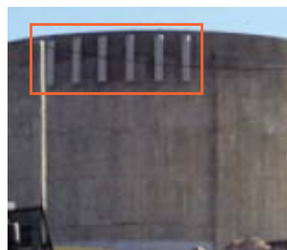
Panel antennas flush mounted on a water tank.
