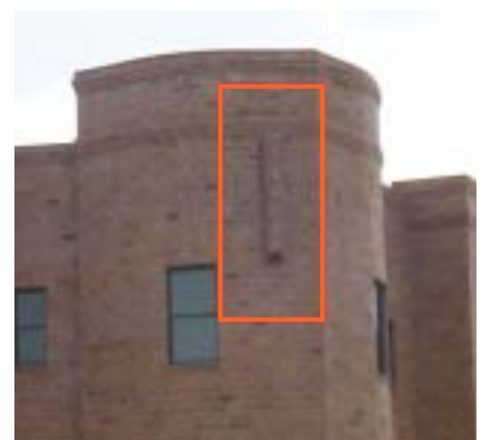
Antenna matched to the brick background on a landmark building.
