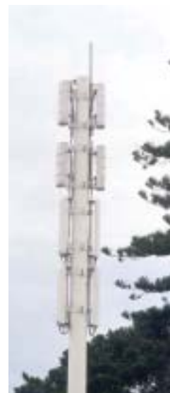
The co-located antennas repeat the form and pattern of the original pole.
