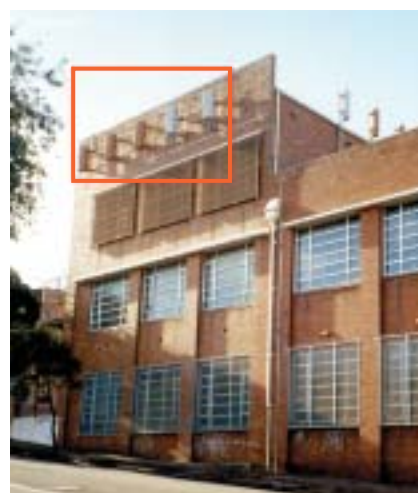
Flush mounted panel antennas. The two on the right have not yet been coloured to match the background.
