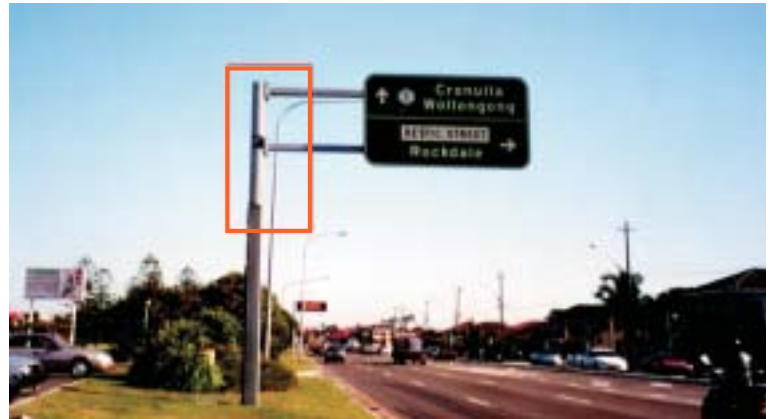
Panel antennas flush mounted to a road sign.
