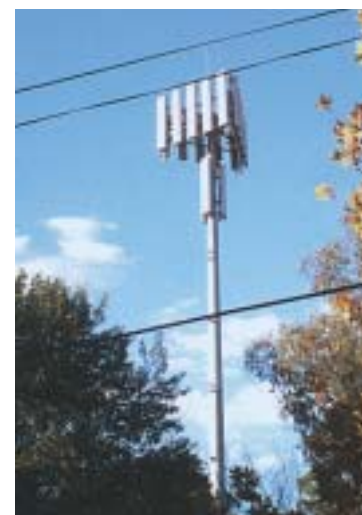
Co-location facility with antennas flush mounted below the original headframe.
