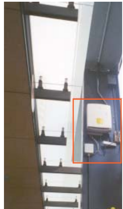
Typical microcell equipment box.
