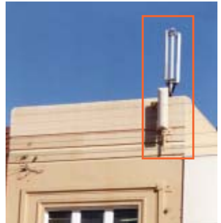
This example illustrates the difference between a flush mounted antenna and protruding antennas mounted near the edge of a building.
