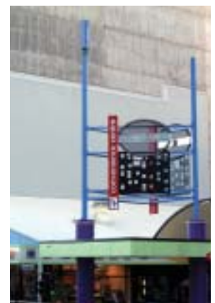
Panel antenna coloured to match the structure to which it is attached.
