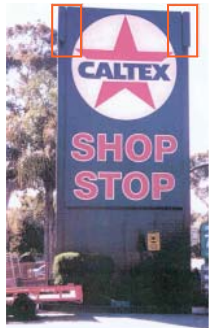
Flush mounted panel antennas carefully matched to the colour of the sign to which they are attached.
