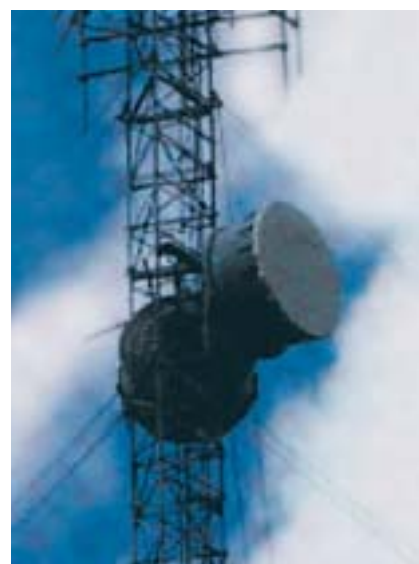
A 1.8m dish, which is low-impact in industrial and rural areas.
