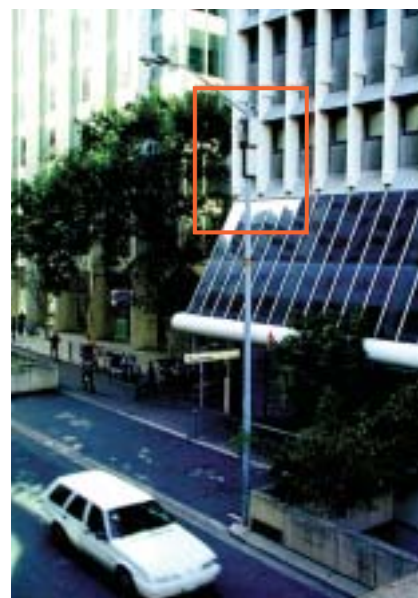
Antennas mounted at the top of a light pole out of the normal line of sight of pedestrians below.
