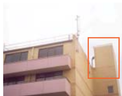
Brick equipment shelter on a rooftop, integrated with the building form.
