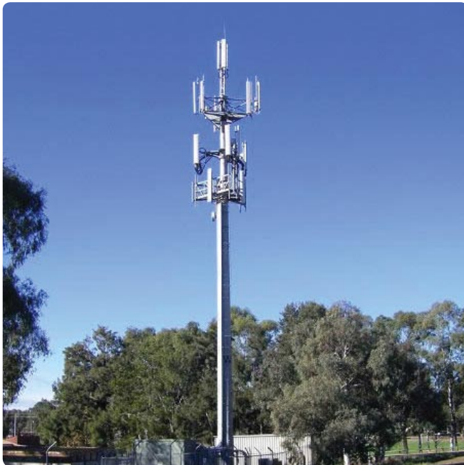
The maximum level of RF emissions from the base station in Holt, ACT, was only 0.127% of the safety standard limit.
